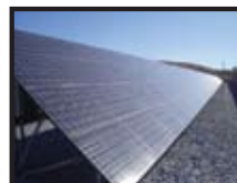
PPL Renewable Energy Park - Camden Co., NJ 500kW System Performing at 105%
